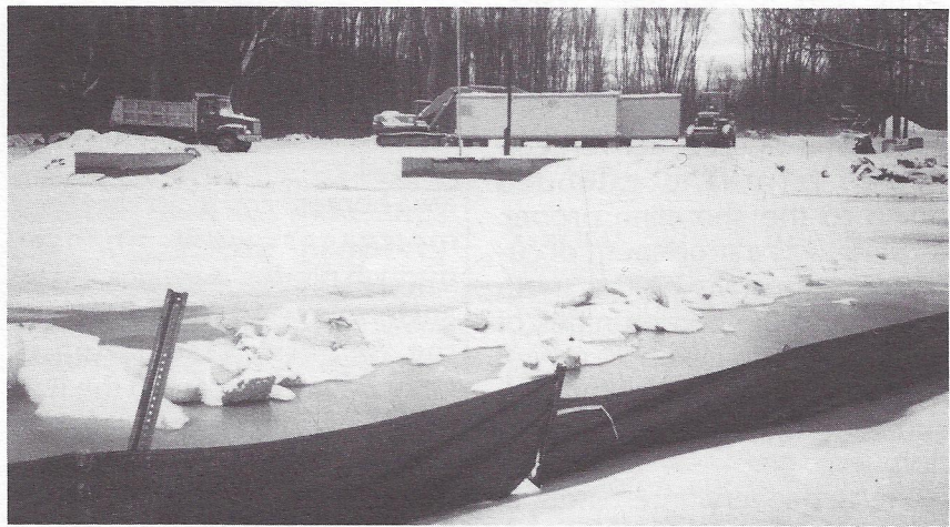
Work being performed for the new Oneida Lake South Shore Boat Launch
